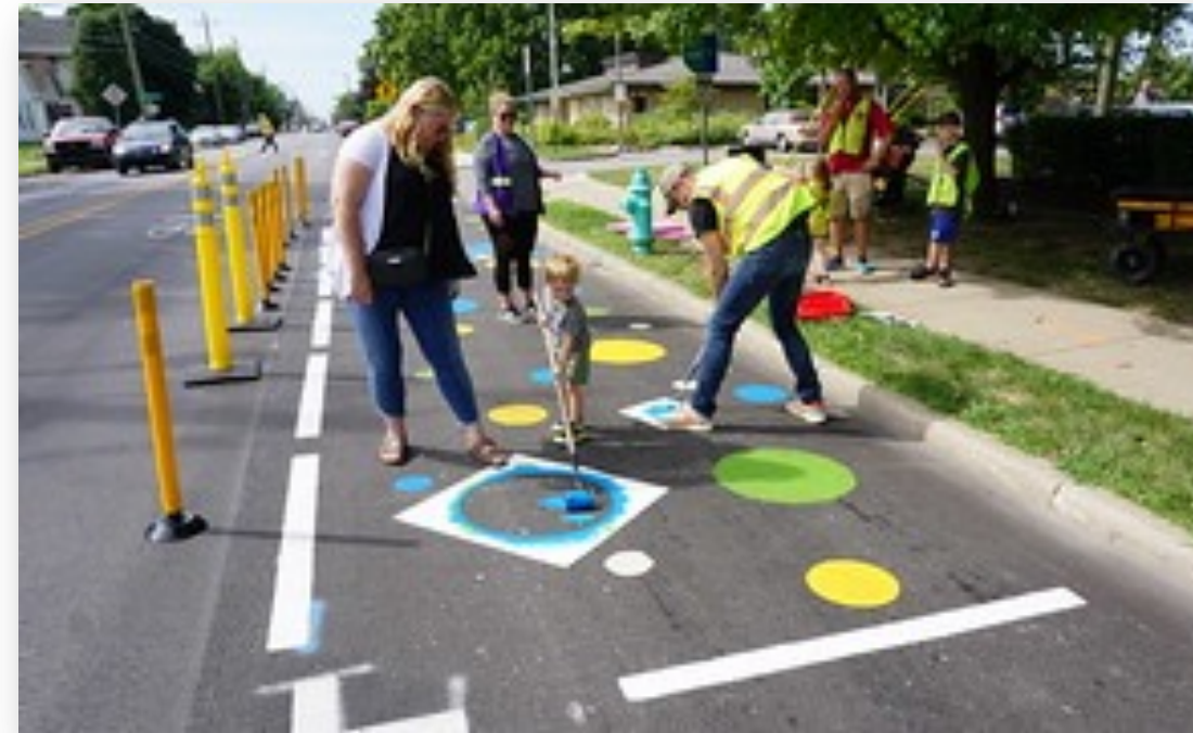
Constructing a bumpout as part of a tactical urbanism project (Big Car Collaborative)
